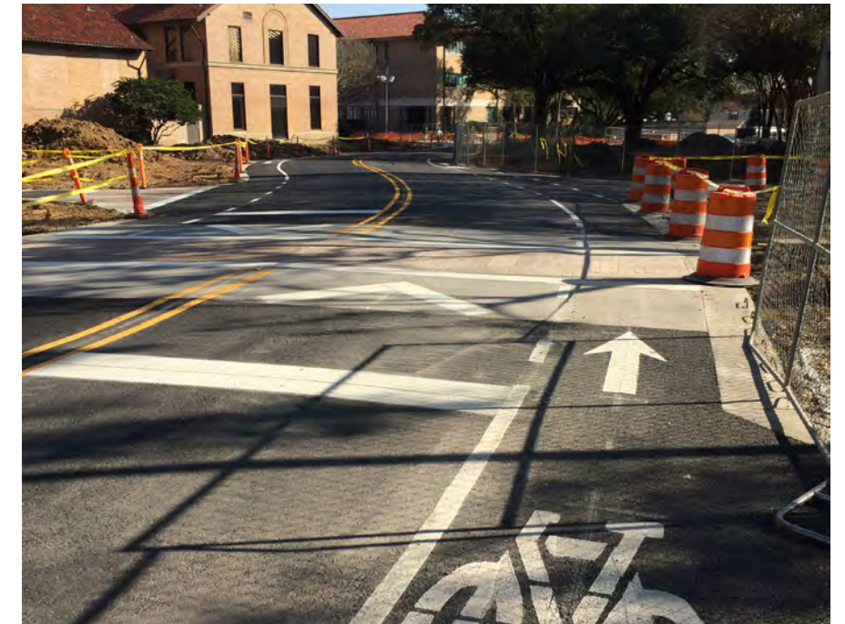
INTERVENTIONS ON FIELDHOUSE DRIVE HAVE SET THE STAGE FOR COMPREHENSIVELY RETHINKING HOW RIGHT-OF-WAY IS SHARED
